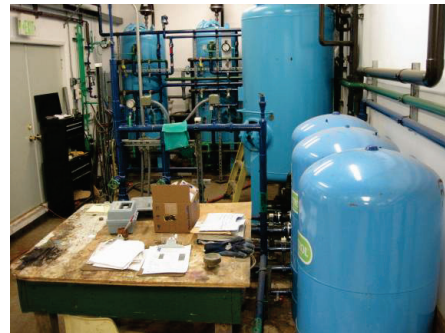
Water Storage and Treatment Tanks
