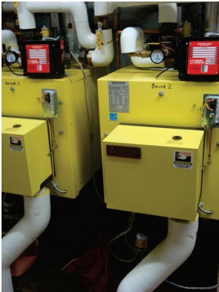
New Energy Kinetics Boilers
