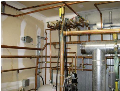
Uninsulated Hydronic Piping System
