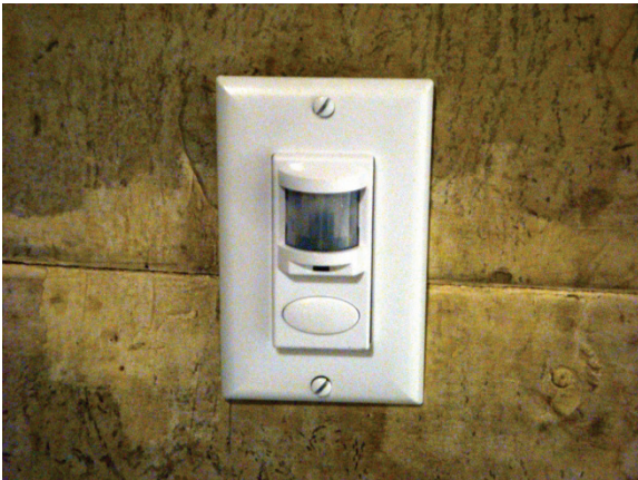
Installed Occupancy Sensor
