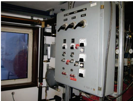
Lift Station Panel
