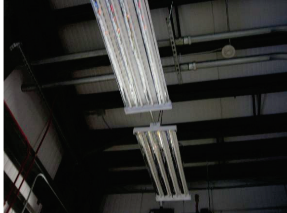
High-Bay Lighting System
