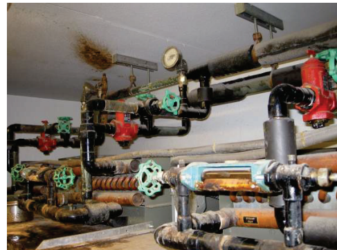
Hydronic Heating System for Dryers
